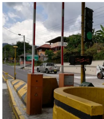
Fig. 2.4. Barrera Vehicular Automatic System BL229
