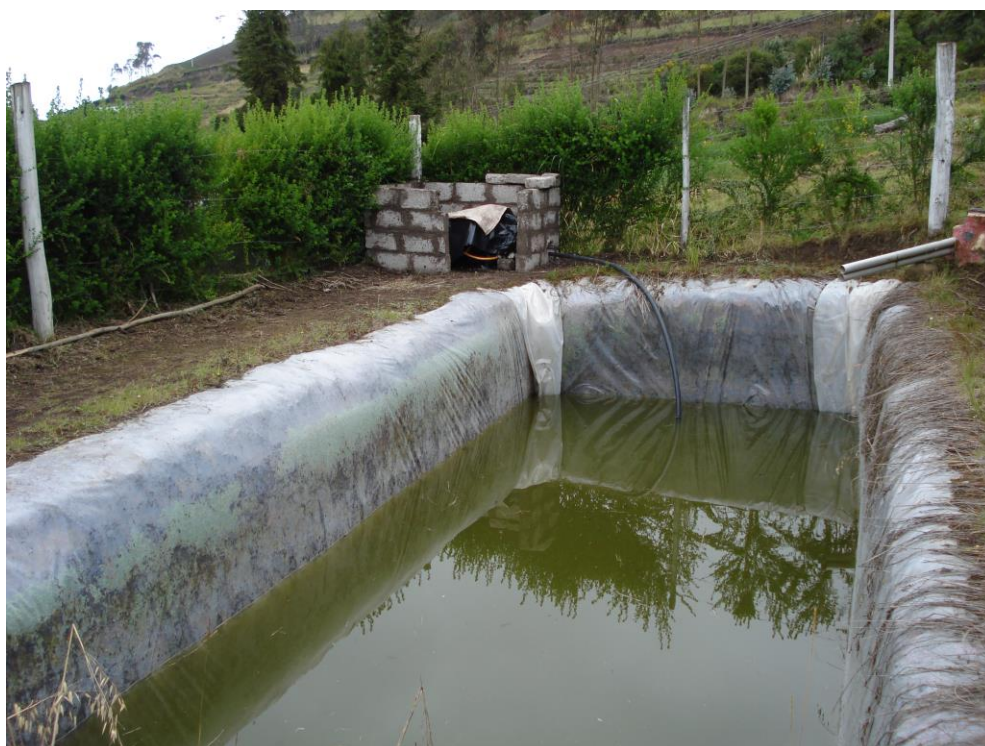
Tanque reservorio individual
