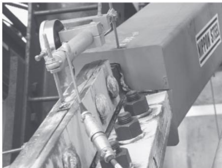
(c) Buckling at brace end
