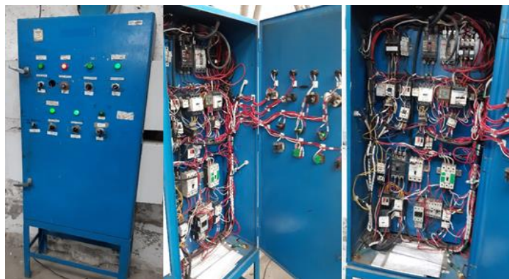
Figura 21: Tablero Control de Bombas
