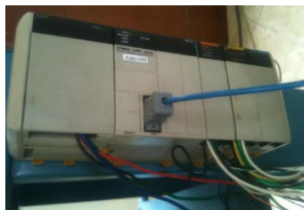
Figura 6.15: Sysmac PLC CQM1
