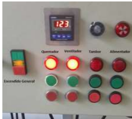
Figura 6.11: Panel de control general
