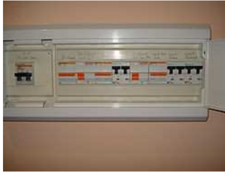
[Figura #47]: Interruptor diferencial 41
