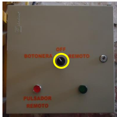
Figura 3.149 Tablero de control
