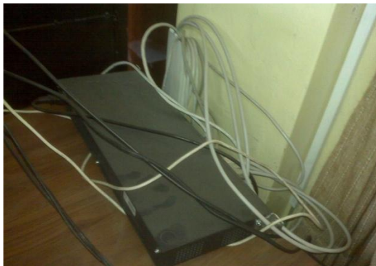
Fig. 1A-9 Switch 3COM 24 Port
